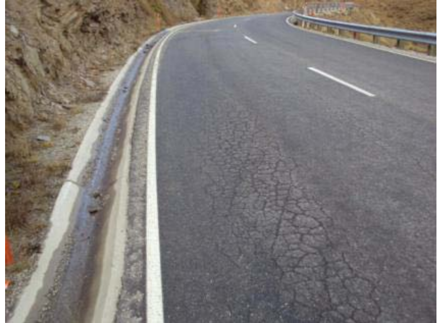
Isolated alligator cracking of asphalt on Crown range FBS site.
