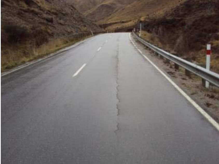
Longitudinal Cracking in Asphalt on Crown Range FBS site.
